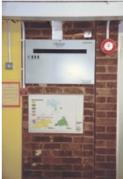
Fire alarm panel, zone plan, break glass call point and fire bell
